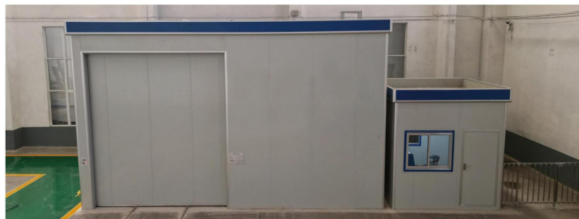
Partial discharge test
