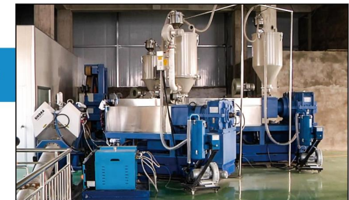
MV Cable Workshop
